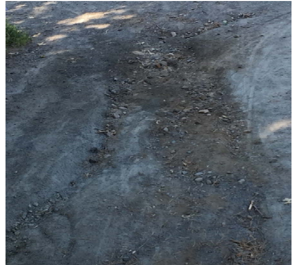
Figure 9 Rutting in the trail surface from drainage problems
