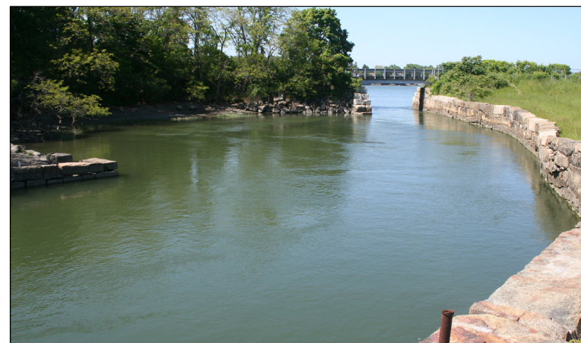
Tide entering the Forest River from Salem Harbor. At high tide the water is only a few feet below the top of the wall. During a large storm this wall could potentially be breached.
