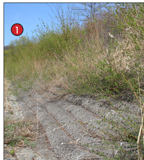
Fiber mats tucked into the embankment and planted to stabilize the slope.
