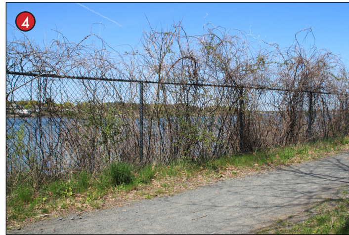
Along The Path views are blocked by a chain link fence that also restricts access down the unstable beach embankment.
