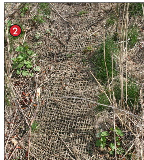
Patches of fiber are exposed due to erosion and lack of vegetation.
